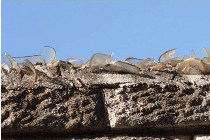
Broken pieces of glass cemented on the wall To prevent football fans from climbing over the wall
